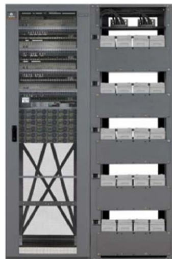
48V Battery Rack with NetSure™ 7100 DC Power System
